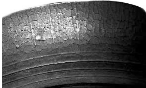
Sidewall Cracking Figure 310
